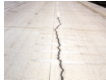
Stitched longitudinal joint and crack.
