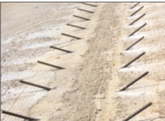
5. Inserting bars into prepared holes containing epoxy. (Note: The bars shown here are in position but not fully inserted.)
