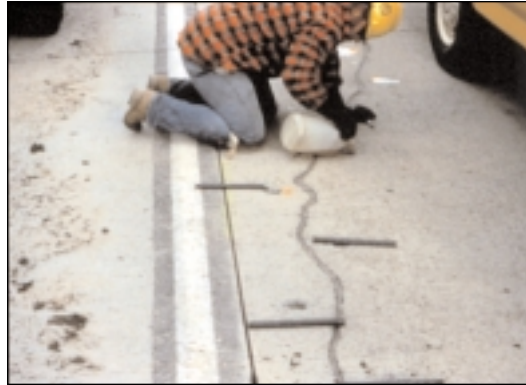
4. Pouring epoxy into drilled holes. (Injecting epoxy is preferable for large quantities.)
