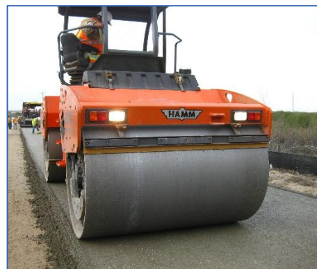
(Right) Equipment operator compacts the RCC pavement with a tandem compaction roller.
