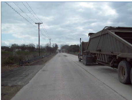
(Above) A truck travels along the completed section of RCC pavement hours after placement.
