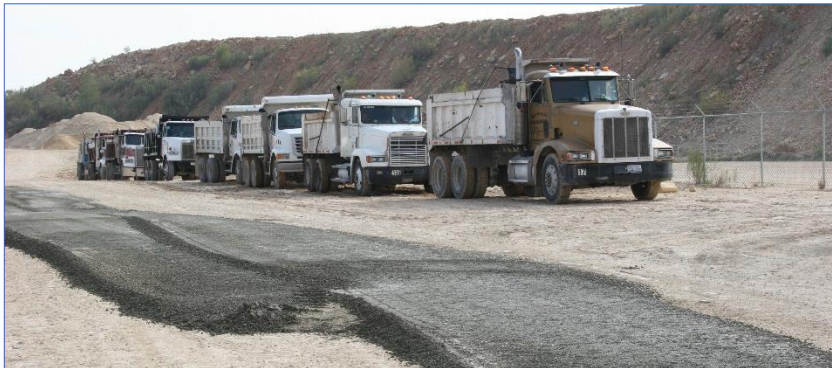
(Left) Photo illustrates the required test strip placed for the project. Placing test strips is considered a best practice for RCC.
